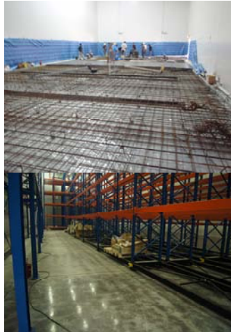
Photos from top: casting of first 2 bays with steel reinforcements & slip membranes in position and Finished floor with mobile racking installed
